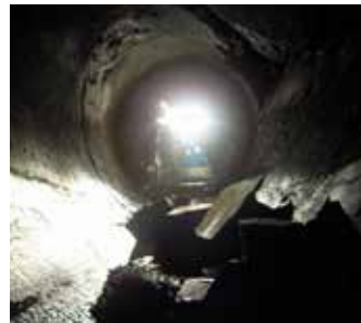
Block fall in the headrace tunnel in 2015, caused by joints and stress induced micro-cracking
