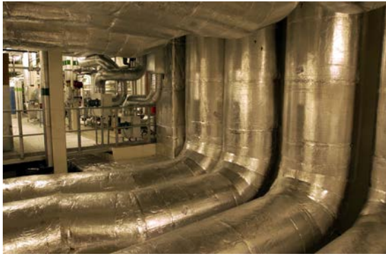
Figure 2. HVAC need space in modern hospitals (Source: HBMN)
