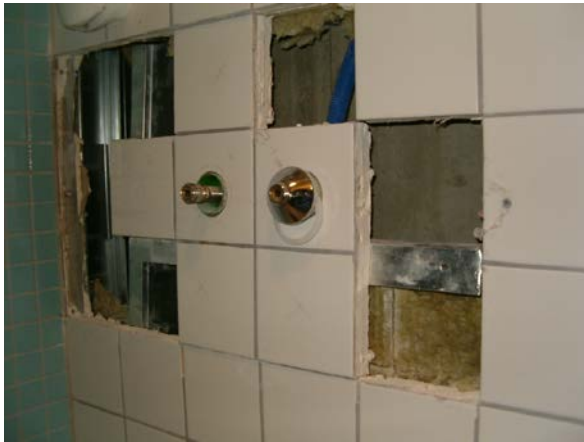
Figure 6. Water leakage in the new bathrooms causes frustrations, delays and money (author's photo)
