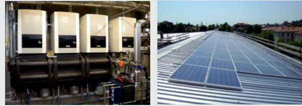
Condensing boiler, photovoltaic panels
