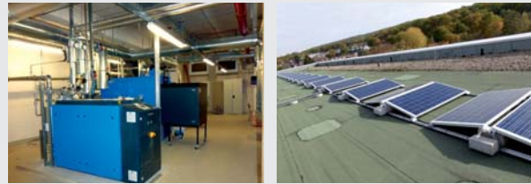
CHP unit, photovoltaic panels
