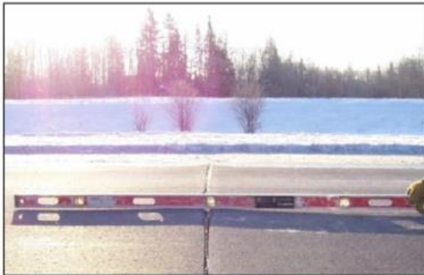
Manual measurement of a tented crack
