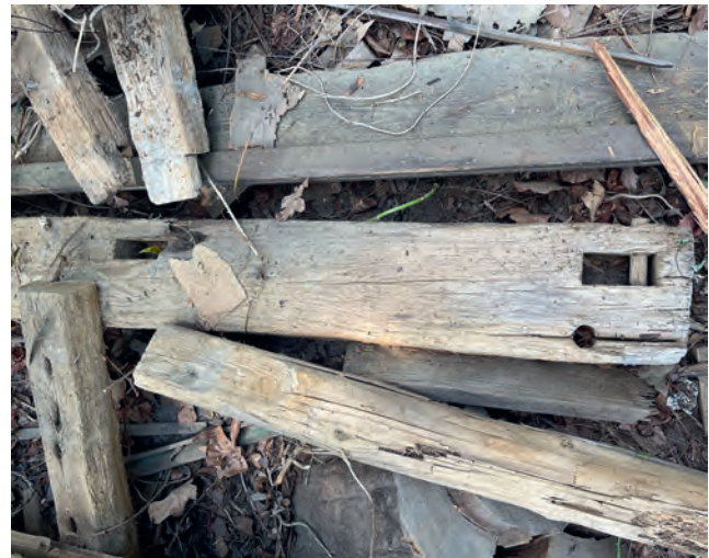
Figure 4. Detail of mortise and tenon in foundation beam and posts. Photo: Christopher Witmore
