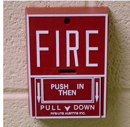
Figure 4: Manual call point for fire alarm system (Schumin, 2002).
