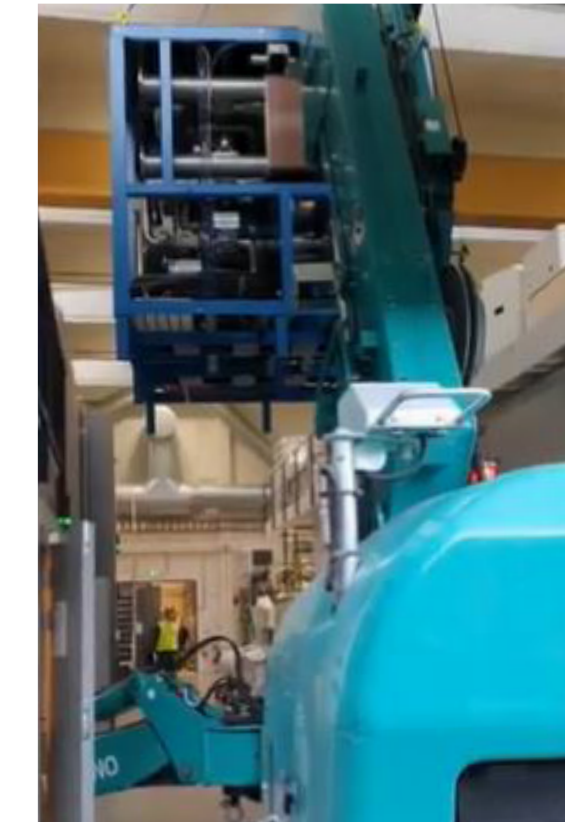
A rare kind of crane was needed to lift this extra heavy load inside the lab.
